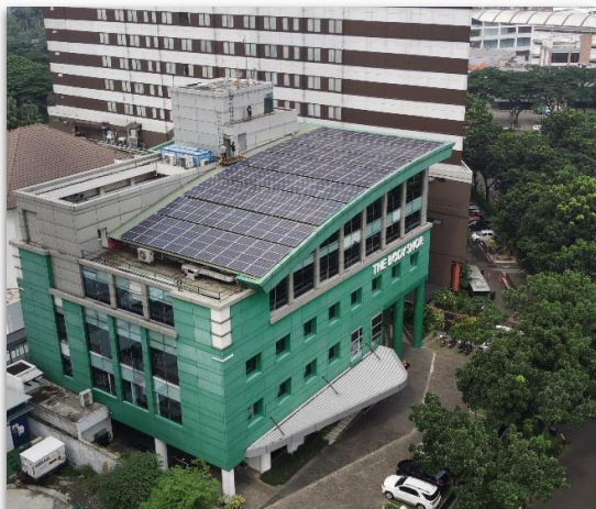
THE BODY SHOP OFFICE BINTARO : 126 kWp
